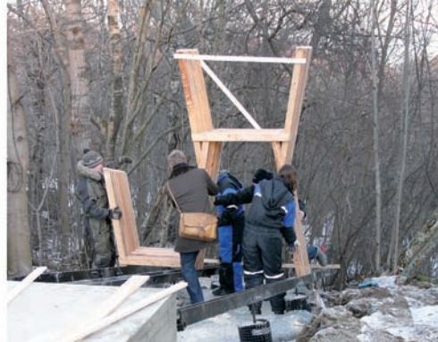
Figure 6 Left, the delivery of the concrete for the foundations; right, the site assembly of a section.
