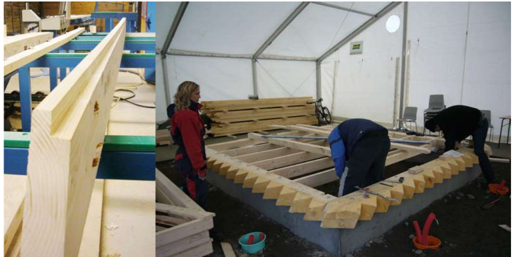
Figure 3 The cut along the wall planks (left) and assembly of the sill beams on concrete foundations (right)
